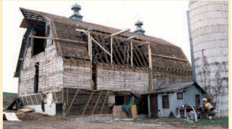
This photo was taken after the original cedar roof and galvanized tin siding had been removed.
