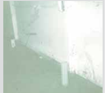
Working inside the barn, Sackett dug a hole next to each post and inserted a pvc pipe, filling it with pea gravel.
