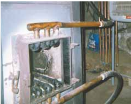
Tim Ojala built this removable hot water booster for his indoor wood stove. Three rows of U-shaped, 3/4-in. brass pipes heat the water.
