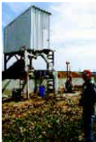
Extruder mounts on stilts in a small shed outside Timmermann's barn. Manure is flushed from the barn into a lagoon and from there it's pumped through underground pipes up to the extruder.
