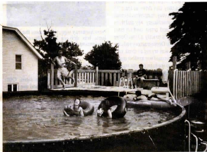
A 20 by 12-ft. deck stands alongside the 4-ft. deep, 24-ft. dia. pool that Beck made from used Harvestore steel silo panels.
