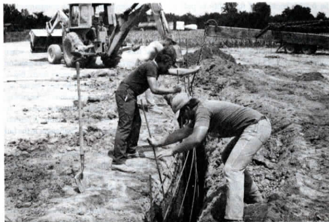
Hass poured the walls of the under-barn manure pit by digging a 12-in. wide circular trench, inserting steel reinforcing rod, and pouring in concrete. After the concrete hardened, he then dug out the center of the pit and poured the floor.
