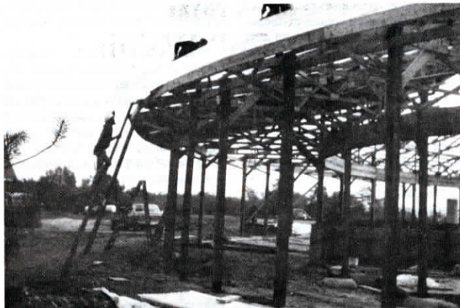
There was less waste than expected in roofing the building because excess steel cut from one edge was used on the other edge of each opposite roof section.
