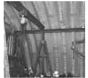
A chain hoist rolls back and forth on the I-beam crossbar.
