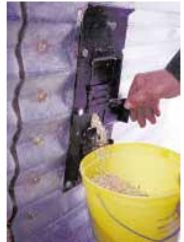
Pipes lead to a “manifold” installed in the outside bin wall. Manifold has three slide gates, one for each pipe.
