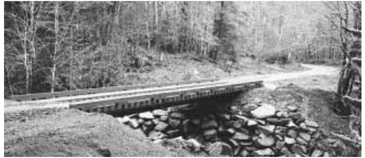
Bridges made from 40, 50, and 89-ft. long flat cars last as long as conventional bridges, says the company promoting the idea.
