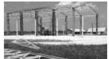
Parts of two old airplane hangars were used in the construction, along with large posts made with beams off railroad bridge.
