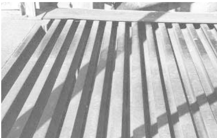
Steel I-beam (not visible) runs crosswise under rails to help support weight of tractors and wagons.
