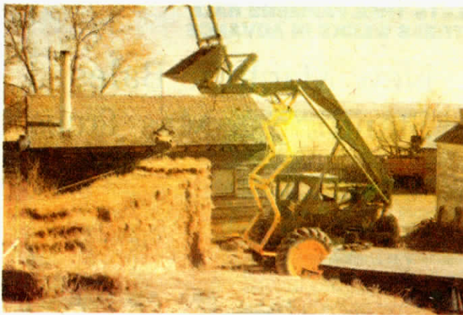
Staffanson used his home-built high-lift loader and "sod forks" to set sod into place for the sidewalls.
