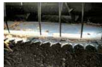
Oakes wrapped 3-in. wide metal clamps at intervals around pipe and bolted them onto platform's frame just behind guards.
