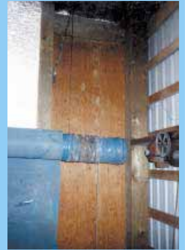
A big plastic pipe attaches to bottom of screens and is raised and lowered by cables operated by a winch and motor.
