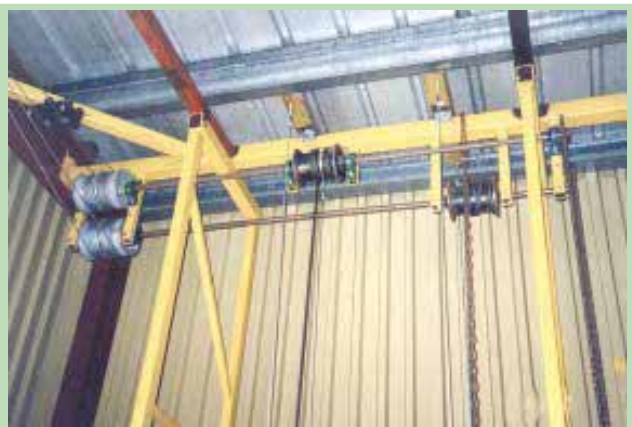
Lift cables run from the bottom of the door to the top and then completely across the width of the building to the opposite corner, where a counter weight frame is located.
