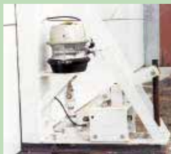
Air brake "pots" are individually plumbed into each end of post to hold it in place. The bottom brake pot shown here is pressurized to force a 2-in. pin into an anchor point in the floor.
