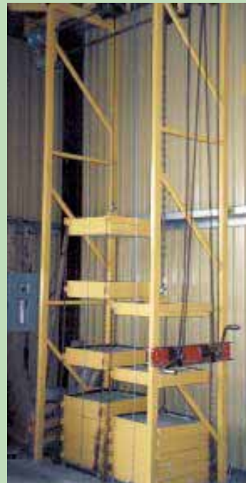
Flat, square counter weights made out of concrete are attached to lift cables. There's one weight per each section of door. Doors are raised and lowered by hand cranks.
