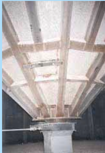
Hopper inside silo stands 12 ft. high.
