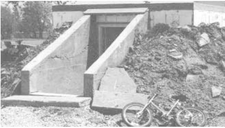
Shelter was built using styrofoam blocks with hollow cores filled with concrete.
