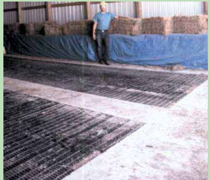
Building has a concrete floor with inset metal grates. Two 50-ft. long, 7-ft. wide tunnels beneath floor bring in warm air delivered by fan.
