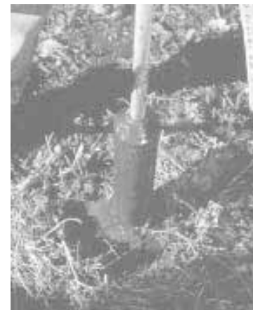
Operator moves tool in a circular motion, then up and down. Water coming out of the tip loosens the dirt and puts it "into solution".
