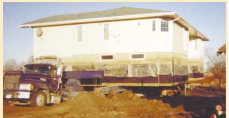
Huyde uses special truck-mounted hydraulic lift jacks to lift both the house's basement footings and sometimes the floor.
