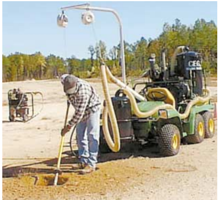
Air-powered shovel uses an air jet nozzle to move dirt. Because there are no sharp edges, it can be used to dig safely around buried power lines and tree roots.
