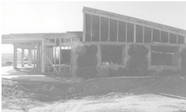
One of the most unusual uses for tire bales so far has been to construct this house for Vernie Houtchens of Pueblo, Colorado.
