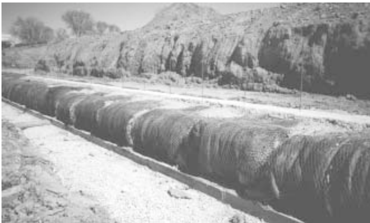
Once compressed, tire bales are held together with five 9-gauge steel baling wires. In photo, a row of bales is being covered with concrete.
