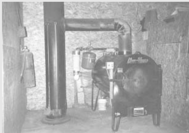
Smoke from stove exits through a steel chimney that extends through shop's metal roof. Switzer mounted a metal catch pan at ceiling level to serve as a rain-proof seal.
