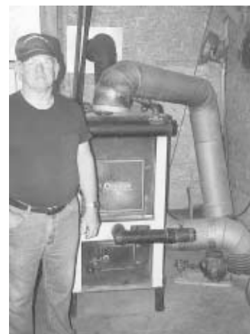
Dale Denton uses underground pipe to carry heat from the forced air furnace in his shop to his house. He buried two lengths of 12-in. field drainage tile 4 ft. deep. One is for hot air and the other for cold air return.
