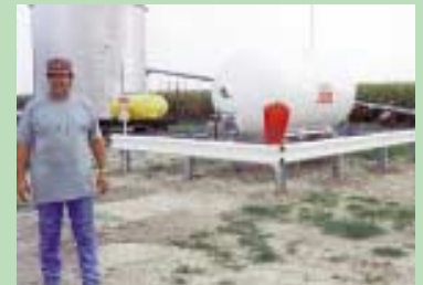
Roger and Bruce Elliott put a complete guard rail around a newly-installed 2,500-gal. propane tank.
