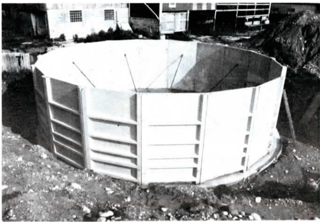
This 12-ft. high tank was built out of concrete panels connected by a patented joint sealing system.
