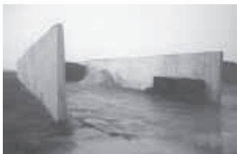
The Martins can pour two or more 30-ft. sections of bunker wall a day. is poured.
