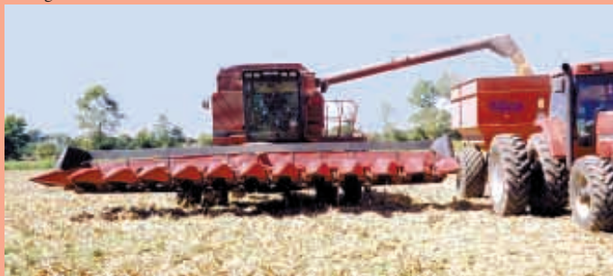
He used steel tubing to build a new frame for the header and bought a new cross auger.
