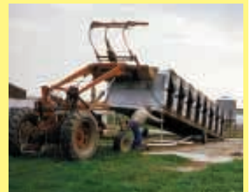
Loader tractor picks up one end of frame, then backs a trailer underneath and pulls it out of the way.
