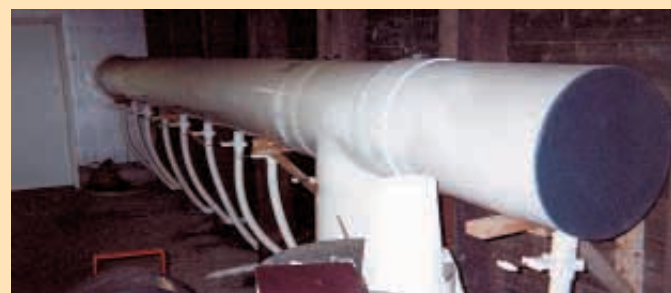
Large air manifold runs down side of building, blowing air into compost.
