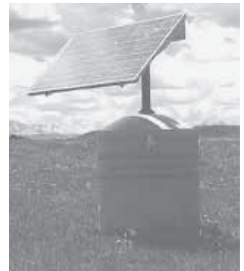
Go-anywhere solar panel sits on top of a “pod” that contains batteries and a DC to AC converter. All you do is install a grounding rod and hook up the batteries. with wind turbines. Thanks to energy rules in Oregon, the owners will receive 18-20¢/KW for power that costs them only 6-7¢ per kilowatt to produce.
