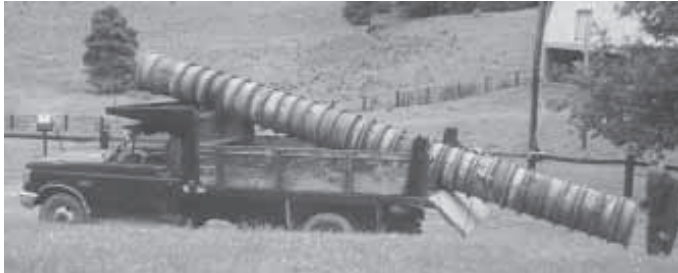
Richard Dunn welds 22-in. dia. truck wheel rims together to form culverts.
