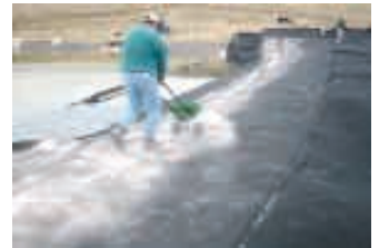
Then a thin layer of Zeolite, a volcanic mineral that absorbs gases, is spread on top of Zeomat with a lawn fertilizer spreader.
