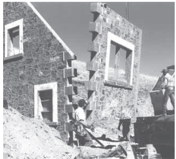
"Tilt-up" stone walls are poured into a form on ground, then put in place with a crane.
