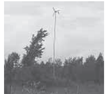
He constructed a 40-ft. steel tower. Blades turn at 210 rpm's and generate 110 volts AC.
