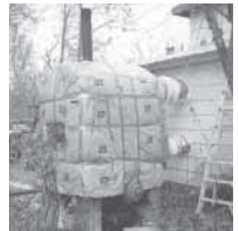
Ackerman insulated stove with 8 in. of fiberglass and ran a metal rod into house so he can work stove's damper from inside.
