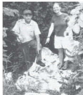
John Nolan has patented his new method for stopping erosion in deep gullies. He uses woven plastic fiber sacks filled with soil.
