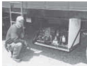
Shelf under bed of truck holds gas engine and blower.
