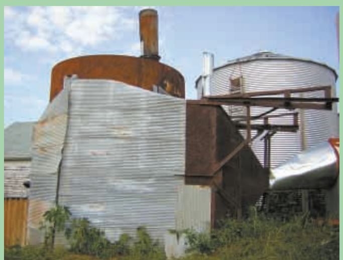
Scrap corrugated tin forms a jacket around the outside of the firebox, capturing heat and directing it to the rear of the firebox where a 12 by 12-ft. hopper acts as a plenum, funneling hot air into the bin.
