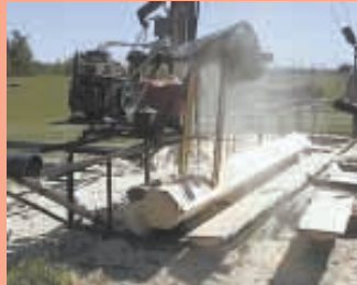
He turns each log four times to cut eight sides. "Octagonal logs produce a warmer cabin because of the increased depth of the joint between logs," says Fraser.
