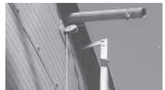
Drain tube from catch pan extends out a hole under roof eave. Steel cable slides in or out of bin.
