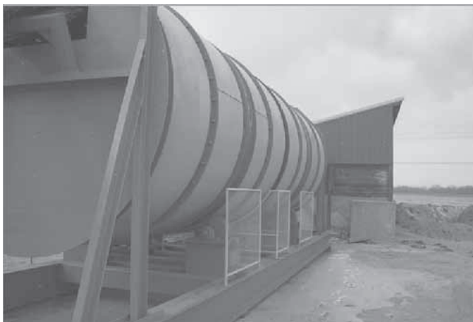
Rotating batch processor takes in manure, garbage, and even livestock carcasses.
