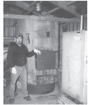
Roger Moore built this outside wood burning furnace out of two old propane tanks.
