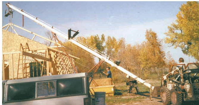
Richard Ackerman converted this 40-ft. long, 8-in. dia. auger into a low-cost crane. "It works great for trimming trees and for lifting rafters onto buildings," he says.
