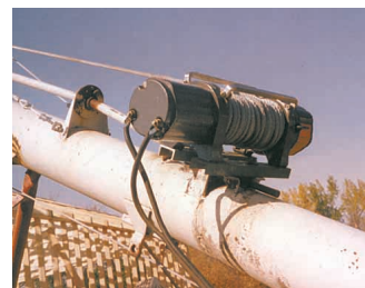
An electric winch with cable was installed on the bracket originally used to hold the auger gearbox.
