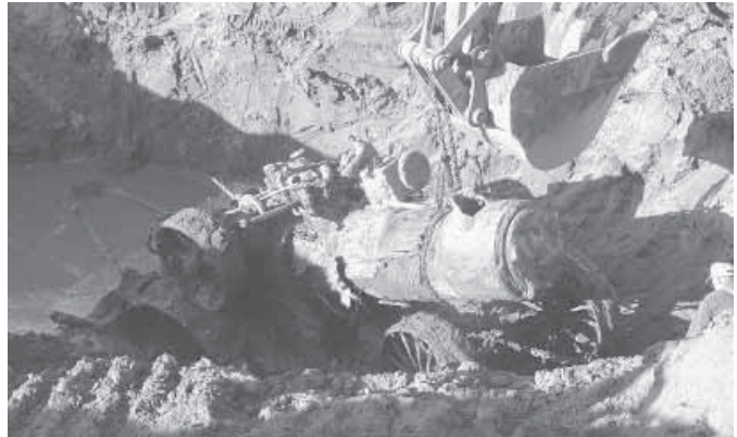
Corey, his father and a crew of buddies with long-handled shovels dug down to wrap a chain around the engine. Then, they used a Cat backhoe and tractor to lug it to the surface, breaking 5 chains in the process.
