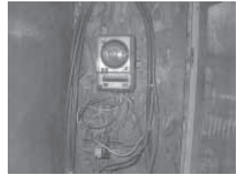
"The timer is just a simple calendar timer that I can reset as day length changes," says Bard. "The opener is an electric motor-driven ball screw. Its threaded shaft screws into a nut on the door."
