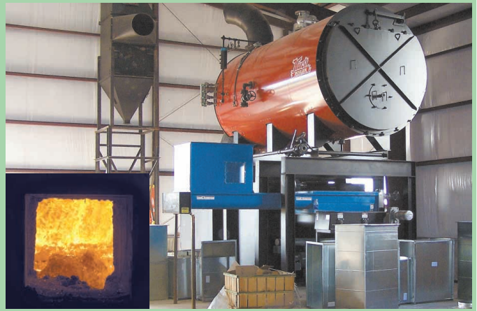
Manure-burning boiler on Wiese Brothers Dairy drives a large electric generator. The extra electricity is sold to a local utility company.
