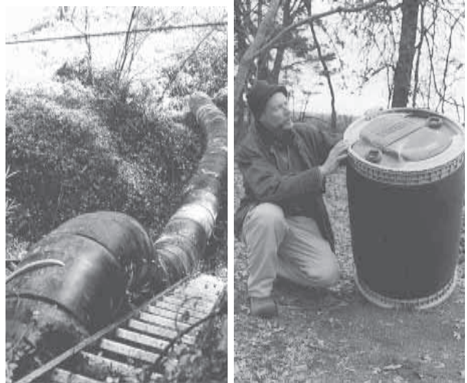
McCann made 150 ft. of large diameter drainage pipe using 55-gal. black plastic drums. Huge pipe snakes down a steep embankment to divert runoff and minimize erosion.
