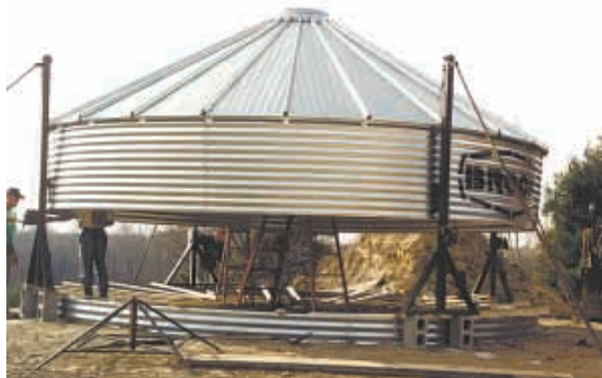
They laid the foundation and poured a floor, then put in two rings of grain bin steel to create 7-ft. basement walls.
