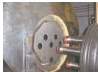
Fans draw hot vapor from floor collectors to insulated ducts, which house a collection of "Isobar" superthermal conductors (left). The Isobars are 3-in. dia., sealed stainless steel tubes containing a proprietary "working fluid". They're inserted into an 800-gal. bulk tank (top) that's filled with water.
